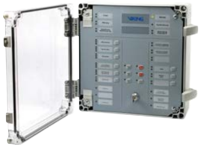
Fire detection and extinguishing control panel
